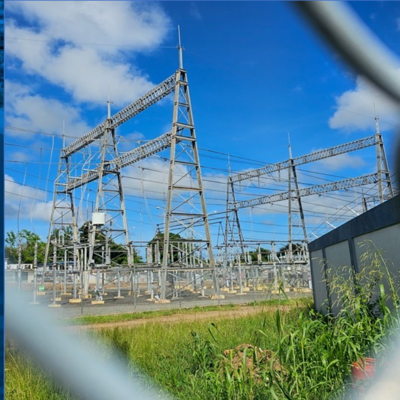
Substation Sabana Llana, Carolina $10 M
