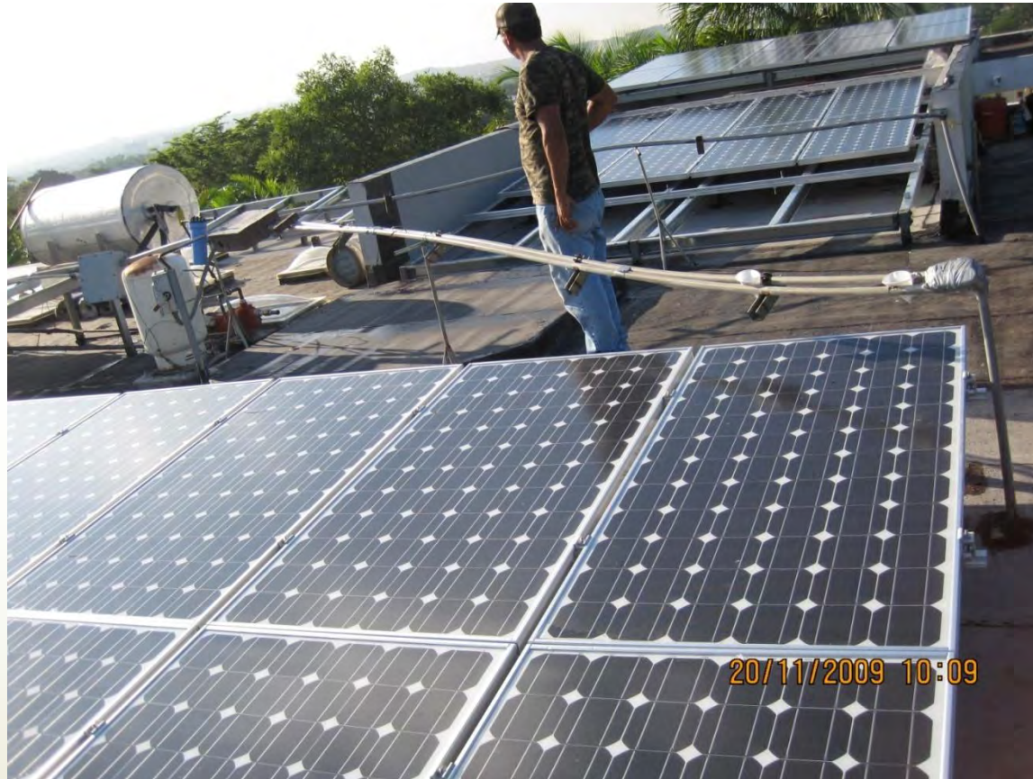
Residential Installation – 8.4 KW
